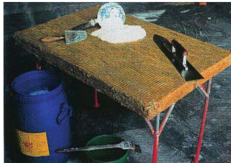
Make up a measuring cup that holds the exact amount necessary to apply the 1.6mm thickness. Pour the coating into the centre of the panel and spread with the trowel.
