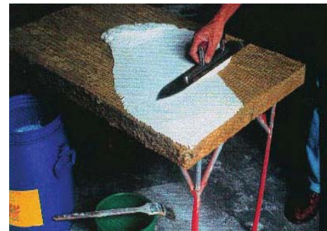
Coat the panels with the KBS Cable Coating by spray or by trowel.
