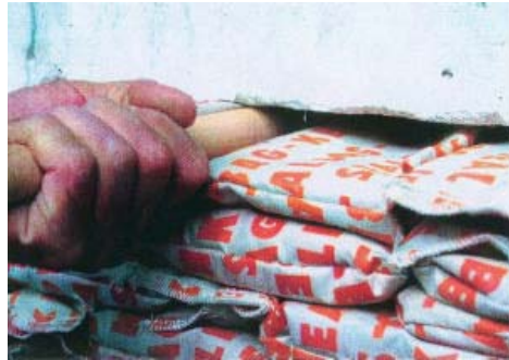
Sealbags being pressed down to seal the penetration before the last Sealbags are installed.
